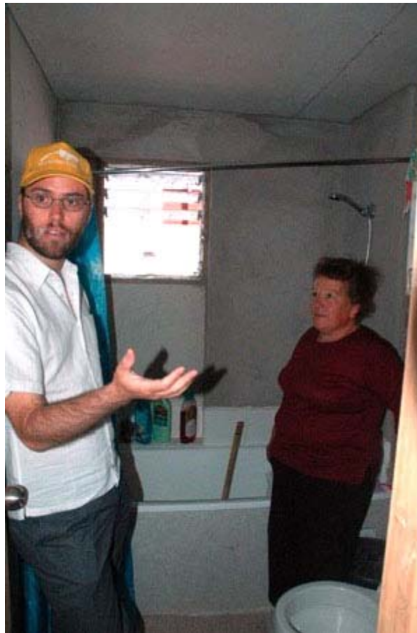
Ortega (right) talks with ELEMENTAL project manager Gonzalo Arteaga in the bathroom of her home. Despite the unfinished walls, residents are pleased that the bathroom in each unit has a bathtub and a window that opens.
